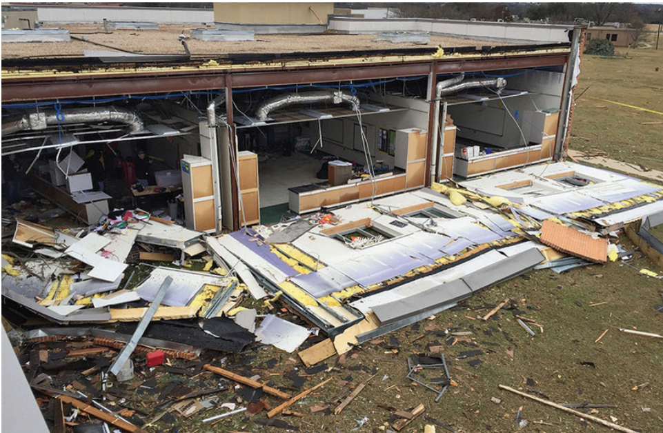
Failing Grades The school may have been more vulnerable to tornado damage because of improper wall-to-foundati connections, including several instances in which, instead of bolts, only small nails were used.
